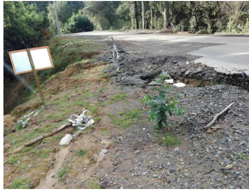
Figure 13: First field visit, lateral view of the slope, detachment from the pavement
